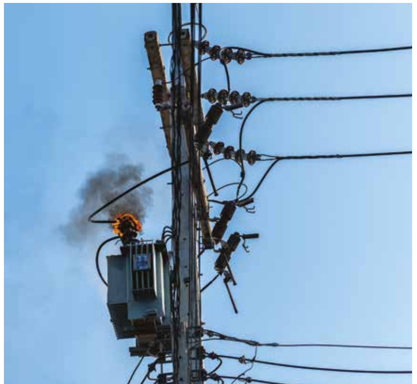
Figure 2. Example of faults in pole-mounted distribution transformers
