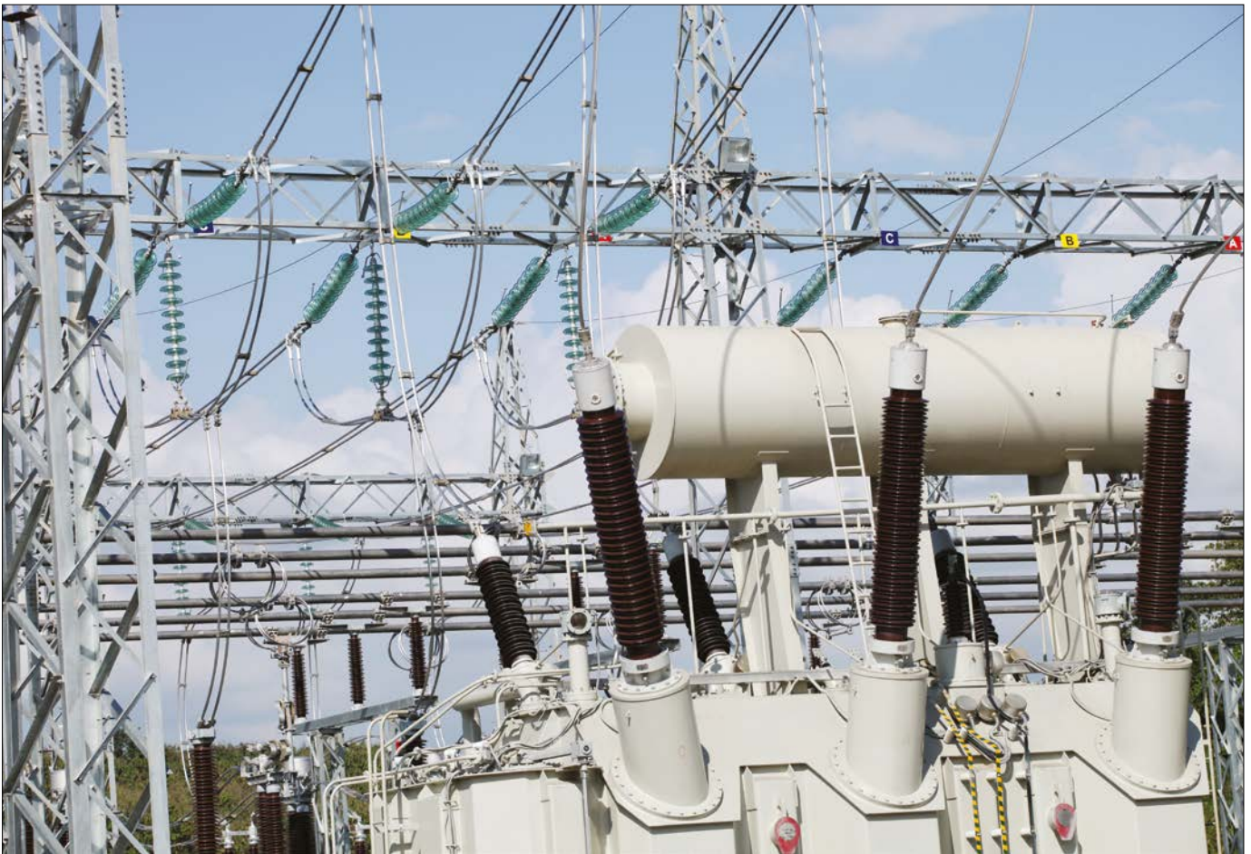
Figure 4. Power transformer bushing
