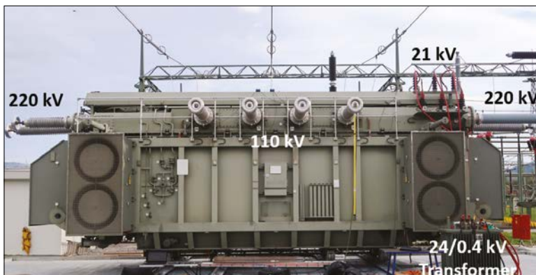
Figure 1. View of the 300 MVA transformer
