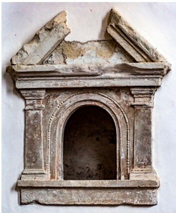
6. Donja Glogovnica, crkva Uznesenja BDM, arhitektonska kustodija na sjevernom zidu svetišta (MKM, KO BJ – F, snimio D. Kirin 2020.) Donja Glogovnica, Church of the Assumption of the Blessed Virgin Mary, architectural custody on the north wall of the sanctuary (MKM, KO BJ – F; D. Kirin, 2020)
