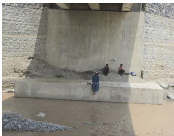
Figure 4 Bridge abutment with exposed foundation due to soil erosion [18]
