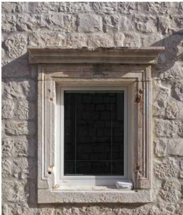
26. Sačuvani sjeverni dio kuće Gattin – Delalle i renesansni prozor na zapadnom pročelju The preserved northern part of the Gattin – Delalle house and a Renaissance window in its western façade
