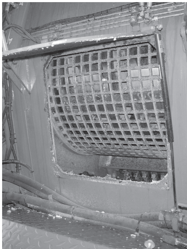
Fig. 2 The screen placed at drum case outlet
