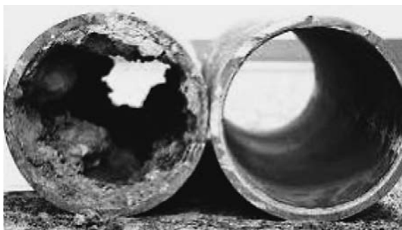
Figure 1 A pipeline fragment with deposits (left) and without them (right)
