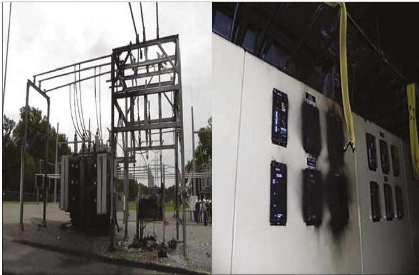
Figure 5. Complete failure of transformer and breaker
