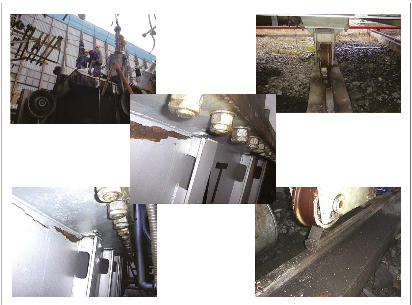
Figures 6. Damage of the 200 MVA autotransformer at S/S “Varna TPP”, Bulgaria
