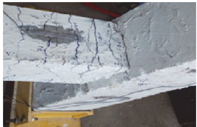
Figure 16. Crack pattern of specimen (S2BRF)
