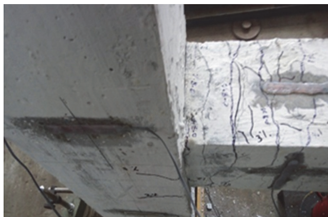
Figure 18. Crack pattern of specimen (S3BRF)
