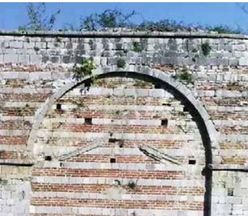
Sl. 20. Sačuvani dijelovi morta krova razorenoga južnog objekta (ispis slike iz snimke Terenca Pepe) Fig. 20 Preserved parts of mortar jointing of the roof of the destroyed south building. (Printscreen made from Terenc Pepa's footage.)
