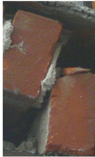
Figure 6. Shearing of the joint between the bricks combined with rotation, photo by Ł. Bednarz
