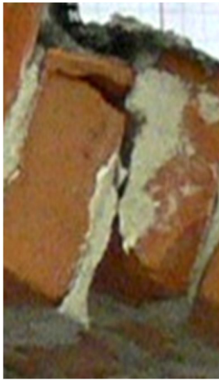
Figure 5. Shearing of the joint between the bricks, photo by Ł. Bednarz
