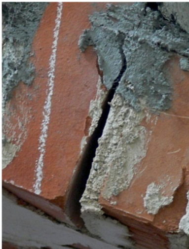
Figure 3. The formation of a joint with a center of rotation in the upper part of the joint, photo by Ł. Bednarz
