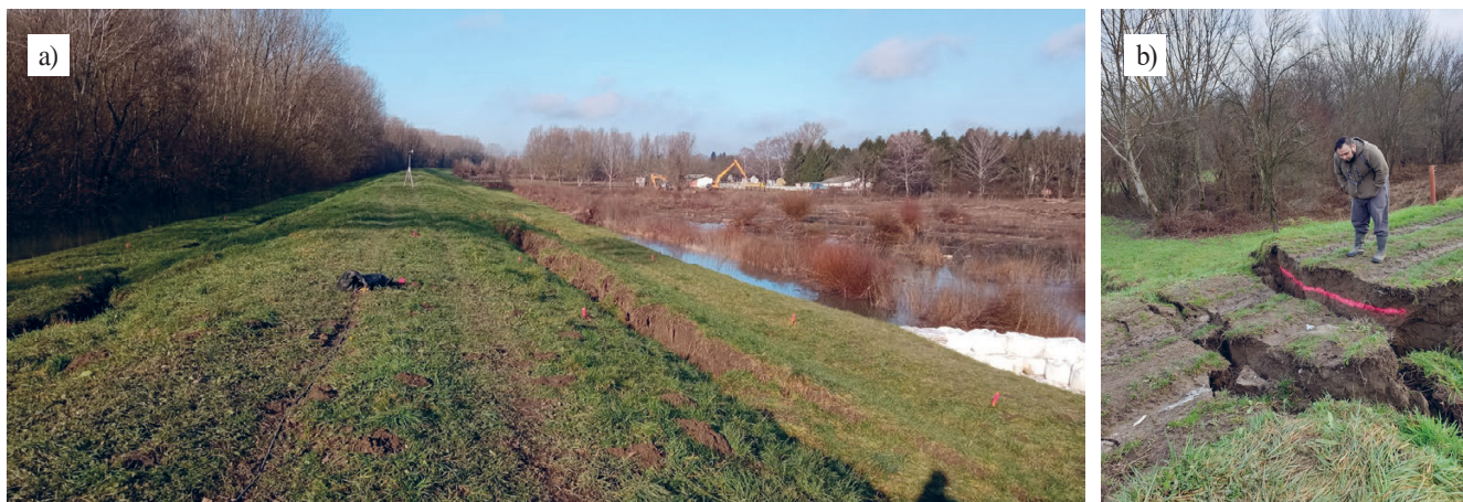
Figure 7. Subsidence and lateral spreading of the embankments near the Sava river: a) in Sisak (observation point Si-03); b) in Palanjek (observation point NP-21).
