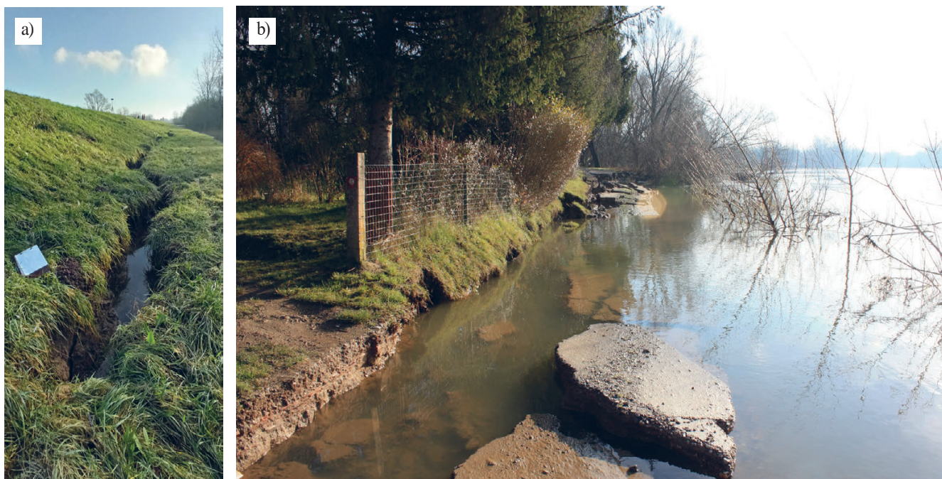
Figure 6. Lateral spreading and associated processes: a) failure of the flood embankment in Sisak (observation point Si-03); b) road failure in Letovanić (observation point RMT-35).
