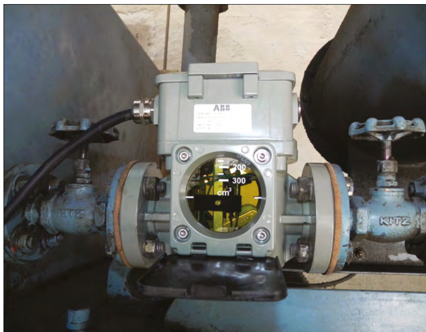
Figure 7. Buchholz relay with two valves. At normal operation, always open.
