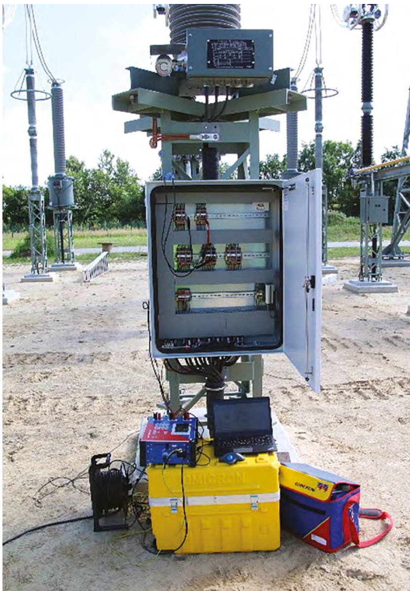
Figure 6. Measuring configuration of the CT Analyzer in the field
