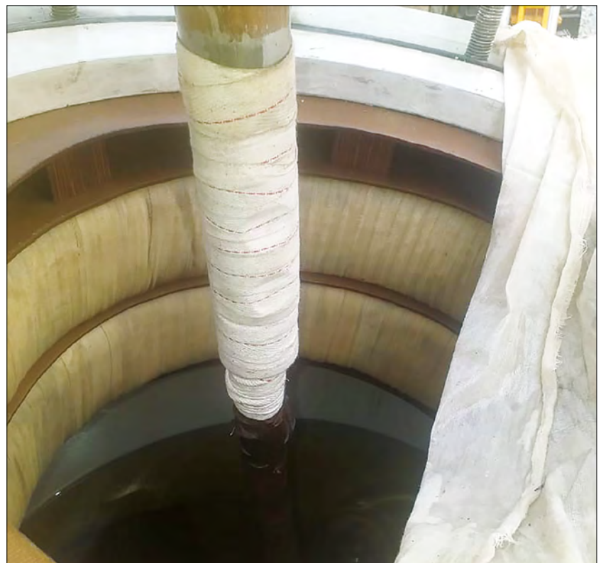
Figure 9. Cotton tape wrapped over the half-lap joints of 1 V phase winding lead and the draw-rod type bushing, tightened
