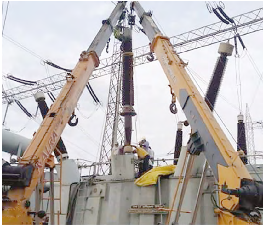
Figure 10. Manoeuvring and lowering down of the TELK’s design 420 kV OIP bushing through 1 V turret of the BHEL’s design 315 MVA transformer with utmost care and precision using two long boom Hydra cranes.
