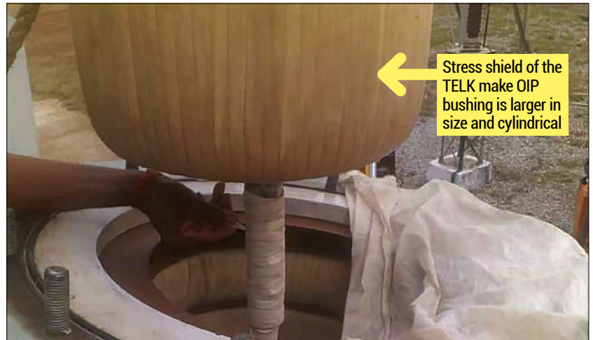
Figure 8. A 420 kV OIP TELK's design bushing being inserted through the turret with a stress shield
