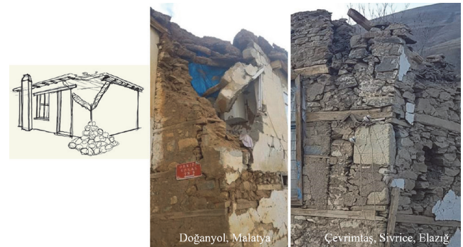
Figure 16. Wedge shaped corner failure
