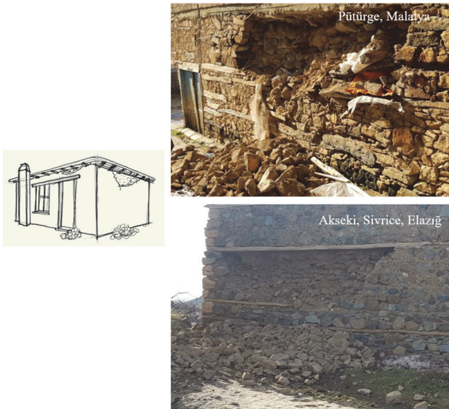
Figure 18. Out-of-plane wall splitting
