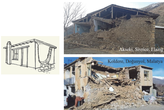
Figure 19. Failure due to wall separation
