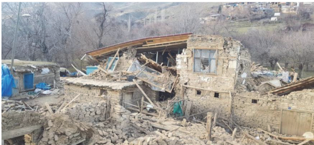
Figure 24. Collapsed masonry building in lower Cevrimtaş village (building 3)
