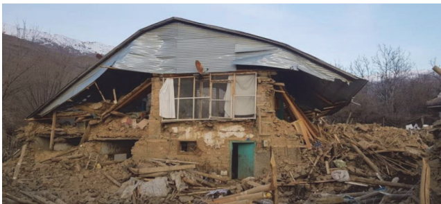
Figure 23. Collapsed masonry building in lower Cevrimtaş village (building 2)
