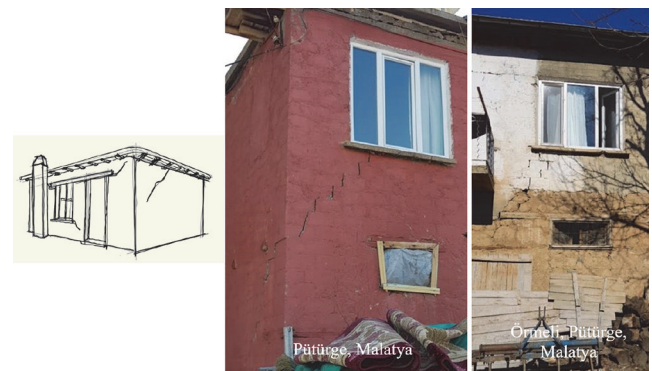
Figure 17. Diagonal cracking on walls
