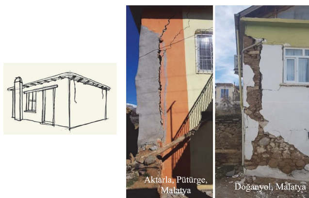
Figure 15. Vertical cracks and splitting at corners
