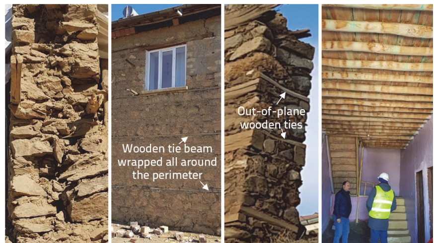
Figure 14. Construction details of typical masonry buildings in the region: a) Wall section; b) wooden tie beams c) out of plane ties d) flooring system
