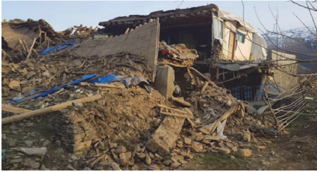
Figure 22. Collapsed masonry building in lower Cevrimtaş village (building 1)
