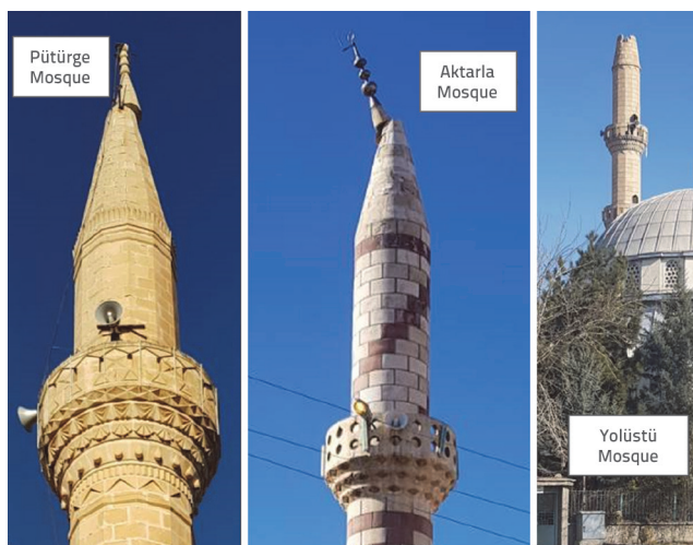
Figure 27. Damage to minarets due to separation of flag from cap
