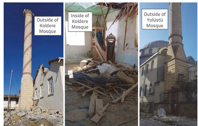
Figure 28. Damage due to falling debris
