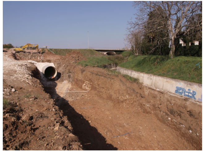
Slika 4. Zidani nosač akvedukta uz desni tok potocića Ričine – pogled na jugoistočni profil unutar recentnog prokopa Figure 4. Masonry pier of the aqueduct next to the right-hand flow of Ričina stream – view of southeastern profile in the recent dig
