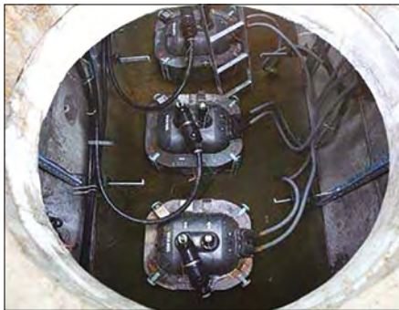
Figure 7. SIDT installed at KEPCO in 2010
