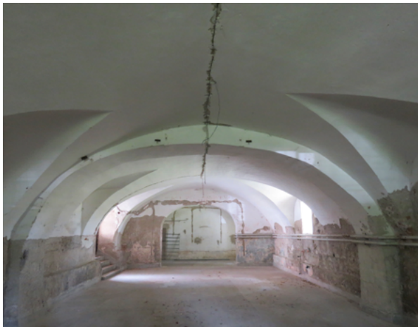
9. Dvorac Kerestinec, bačvasti svod poluukopane prostorije zapadnog krila (snimka: V. Jakaša Borić, 2019.) Kerestinec castle, barrel vault of a half-buried room in the west wing (V. Jakaša Borić, 2019)
