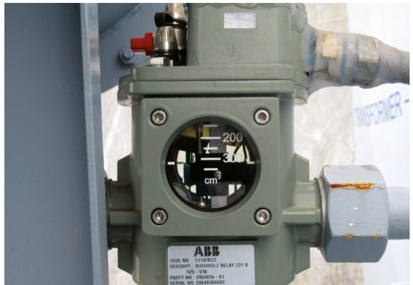
Figure 2. Buchholz relay, the first DGA sensing unit
