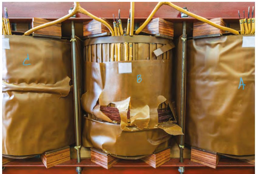
Figure 3. A failed transformer, not deenergized by any trip before the critical event
