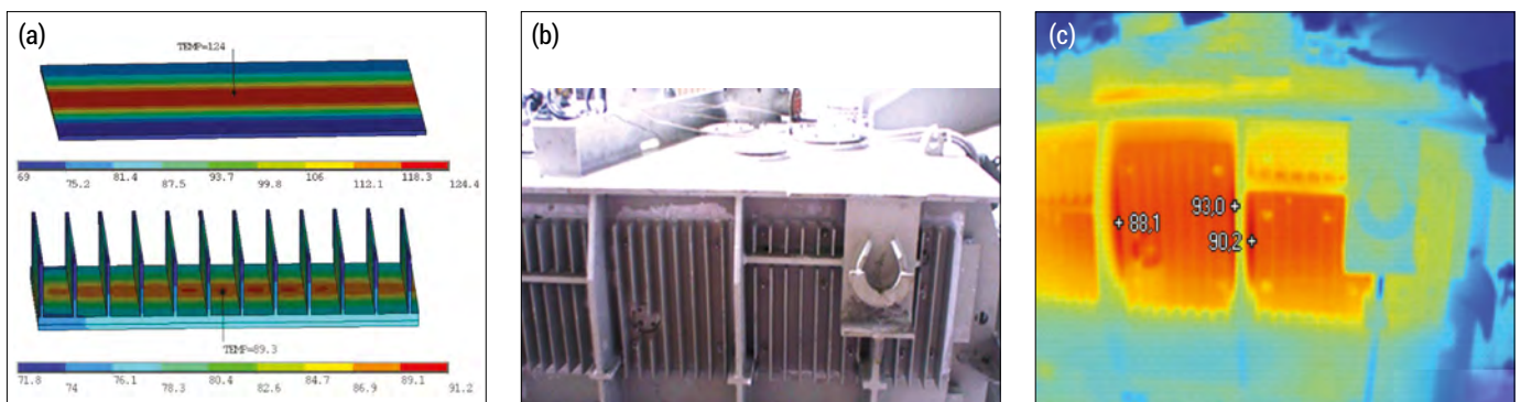
Fig. 6. Reduction of heating of the tank wall of the transformer 45 MVA: (a) – top – basic thermal model of the tank wall part, – bottom – thermal model with a surface-mounted radiator, (b) – installation of surface-mounted radiators on the wall of the transformer tank, (c) – thermogram of the tank wall of a 45 MVA transformer with installed surface-mounted radiators
