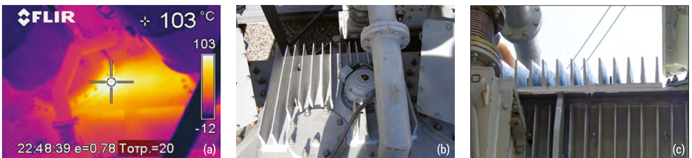
Figure 3. Surface-mounted radiators on the tank of a 200 MVA transformer: (a) – thermogram of the tank cover, (b) – radiator on the tank cover, (c) – radiator on the tank wall
