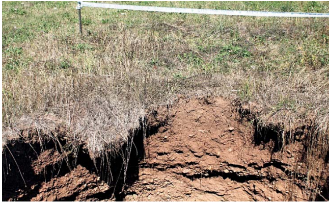
Slika 7. Urušena jama u Mečenčanima, nastala J od ceste, na 2. terasi. Foto. A. Šimunić Picture 7 A Collapse hole in Mečenčani that was formed S of the road, on the 2 nd terrace
