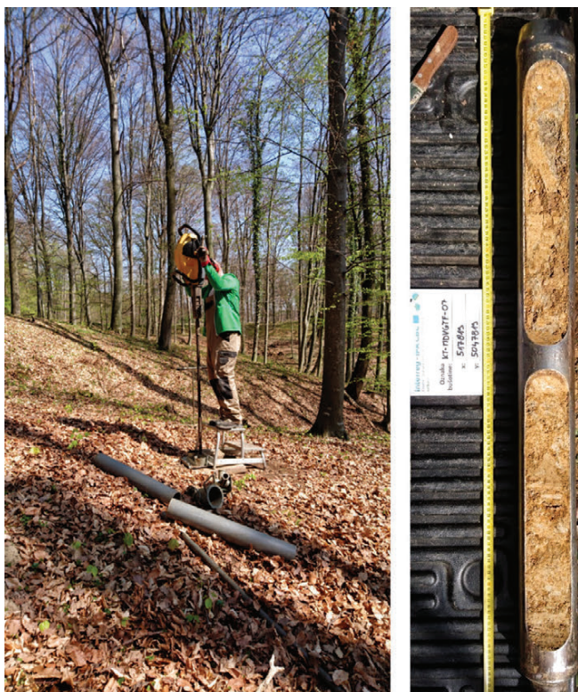
Figure 8. In-situ coring with the Atlas Copco Cobra system and corresponding core. The recovered cores are 100 mm in diameter.
