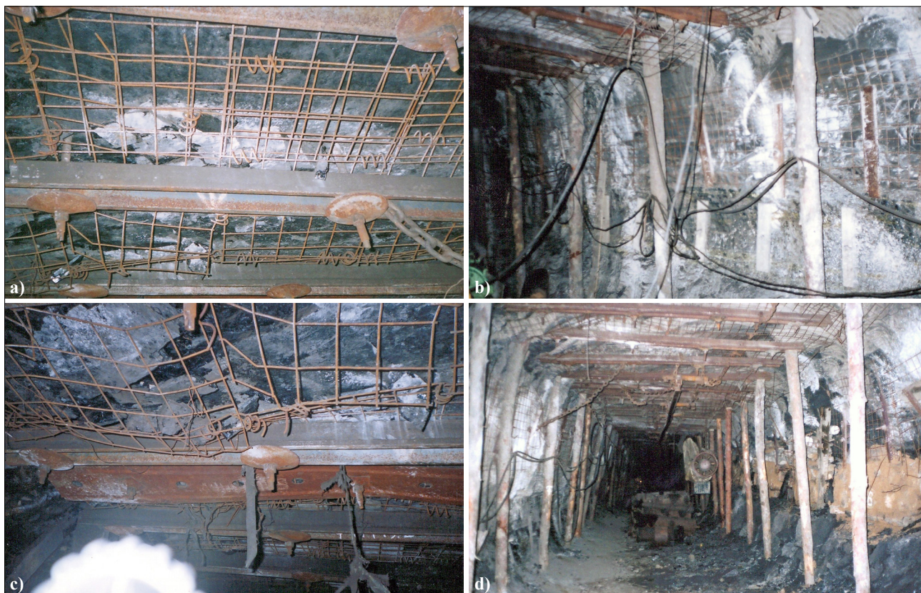
Figure 11. Condition of the rocks of the roof (a, c) and sides (b, d) of the conveyor roadway of the northern main longwall of seam k_5^H at a distance of 25-30 m before the face (a, b) and 25 m after the face (c, d)
