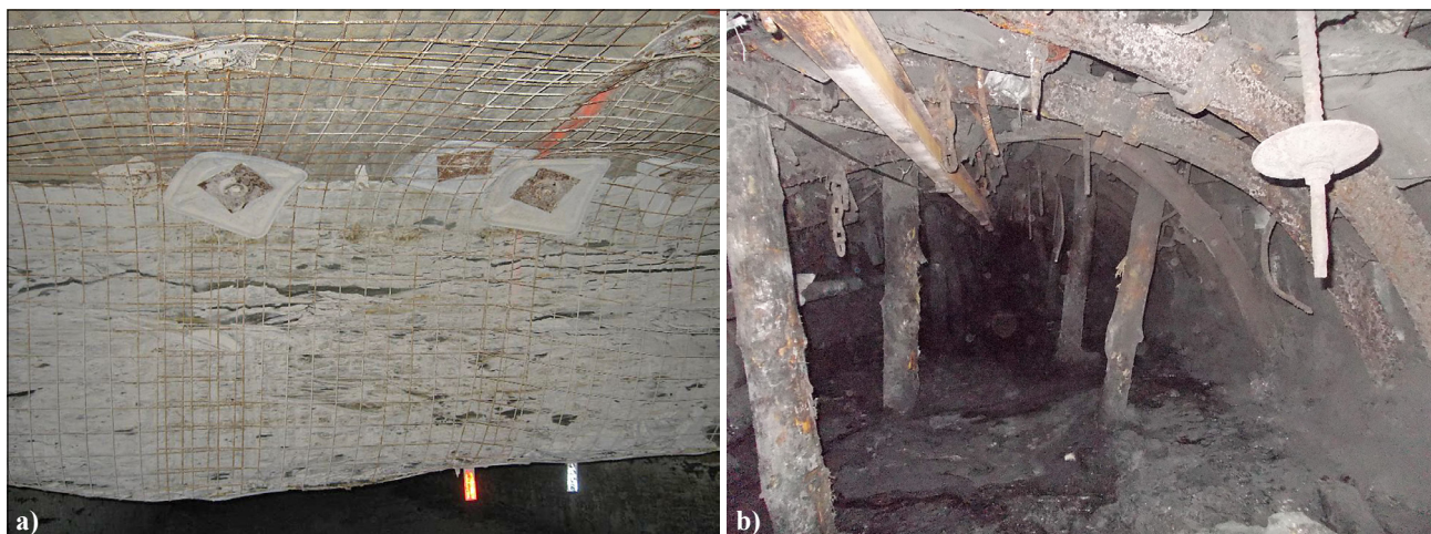
Figure 12. Bed separation in weak shale fixed by rock bolts a) Collections Illinois, USA (Molinda and Mark, 2010) (b) Management Board of the «Pokrowskoje» Mine, Ukraine (authors' photo)
