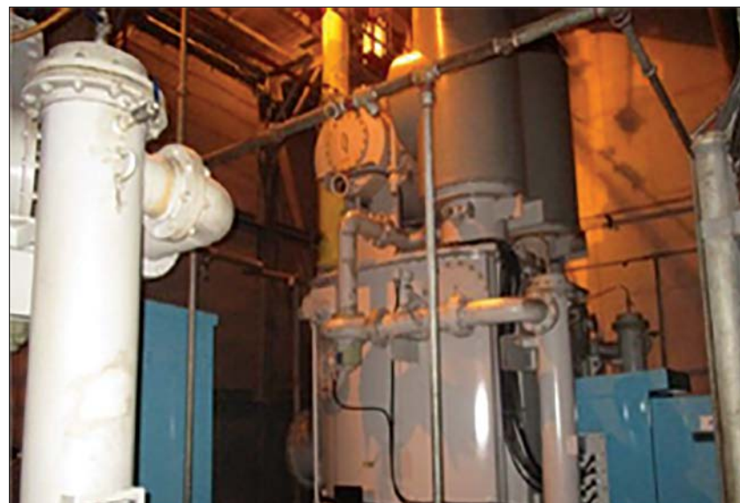
Figure 1. Photo of 90 MVA single-phase GSU transformer
