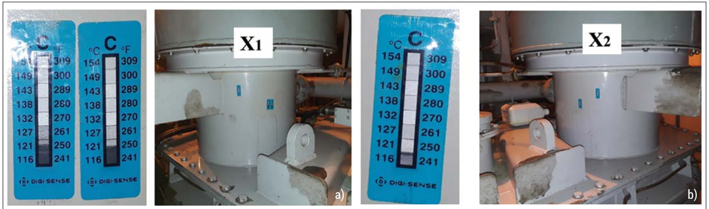
Figure 4. Temperatures measured in the LV turrets with SS inserts at 100 % of nominal current: a) LV turret X 1 , b) LV turret X 2
