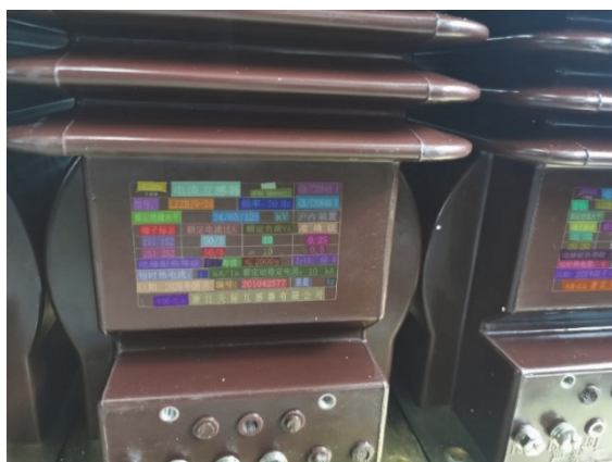
Figure 7 Picture 1 of DBU network transformer detection
