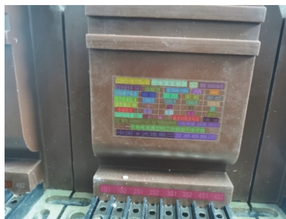
Figure 8 Picture 2 of DBU network transformer detection
