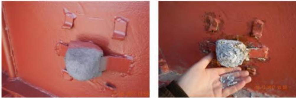
Fig. 2 A sacrificial anode at the beginning of the operation (left) and at the end of its service life (right) [20]
