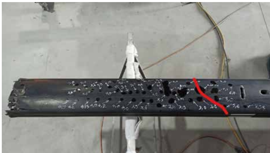
Figure 17 Magnitude of damage 1
