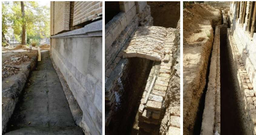
Figure 6 Images of the construction of building No. 4, University of Arts, National garden Campus, Source: (Technical Department and Supervision of Development Plans of the University of Arts) 1400
