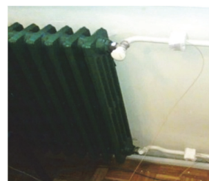
Figure 3 Temperature measurement at supply and return pipes
