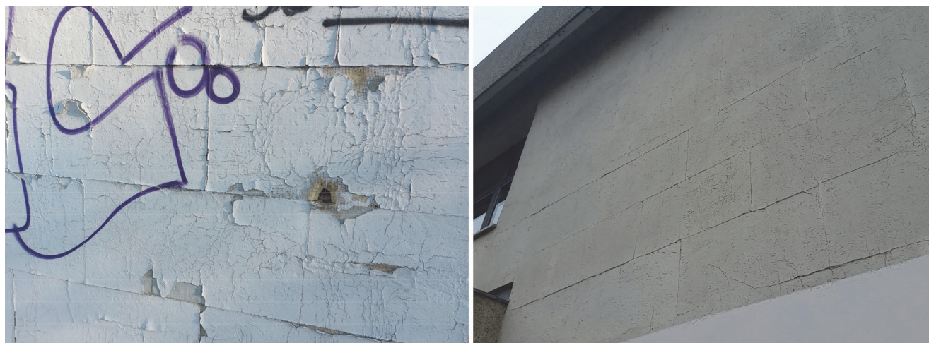
Figure 1. Example of cracked finishing layers of ETICS system due to deformation of EPS boards
