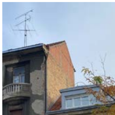
Slika 9 „Saniran“ južni zabatni zida objekta Nazorova 2 Figure 9 "Renovated" south gable wall of the building on Nazorova street 2
