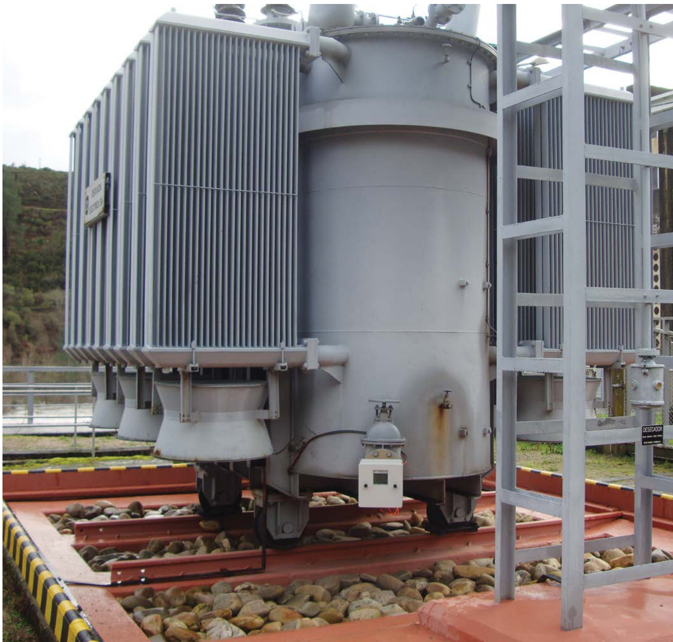
An online device for critical transformers
