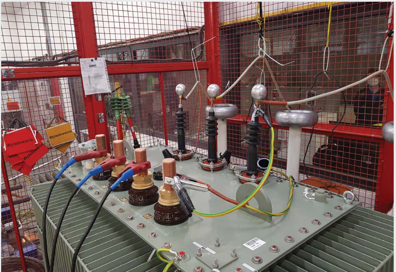
Figure 2. Tested distribution transformer and the setup for the conventional PD measurements
