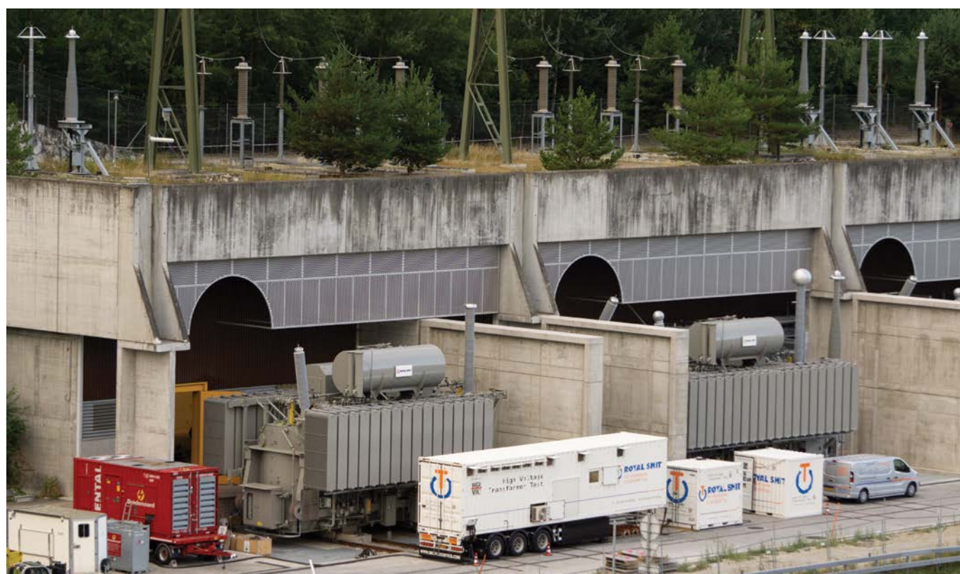
Figure 4. Phase-shifting large power transformers in Swissgrid's transmission grid (photo courtesy of SMIT Transformers)
