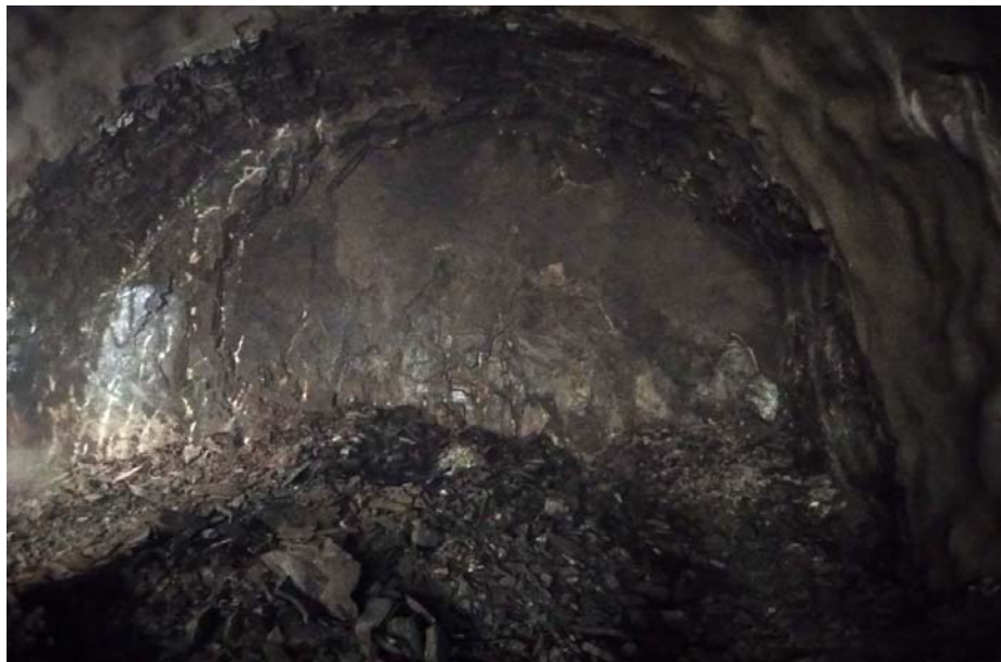
Figure 10. LTT face cross section at chainage 1+524.088 after blasting and treatment of the cross section
