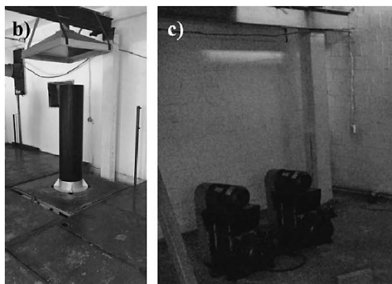
a) - 1st floor, lower part of the column; b) - 2nd floor, upper part of the column with the hood; c) - slurry pumps.
