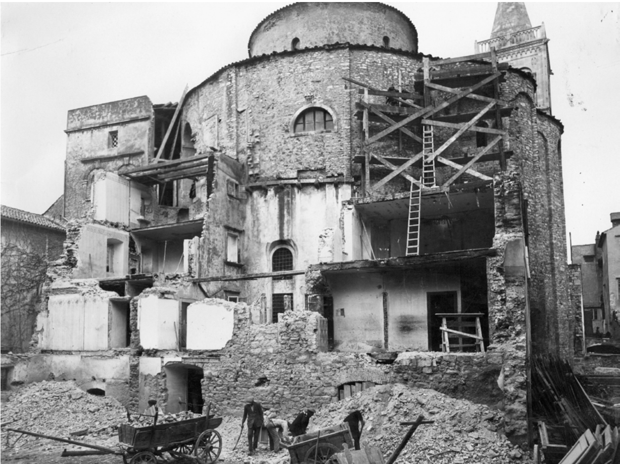
2. Zadar, Saint Donatus during isolation work, around 1930 (Ancona, Soprintendenza archeologia, belle arti e paesaggio delle Marche (SABAP), Photo Archive)
