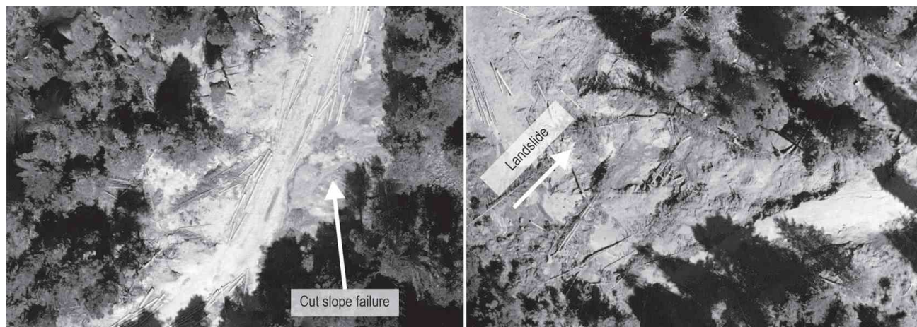
Fig. 5 (Left) Deformation due to lack of culvert at stream crossing of Watershed 8; (Right) Deformation due to insufficient CSA of Culvert 13. The logs in left figure were harvested for road construction but could not be transported as a consequence of road closure due to deformations on road platform. In the right figure, the fall of trees was due to the landslide
