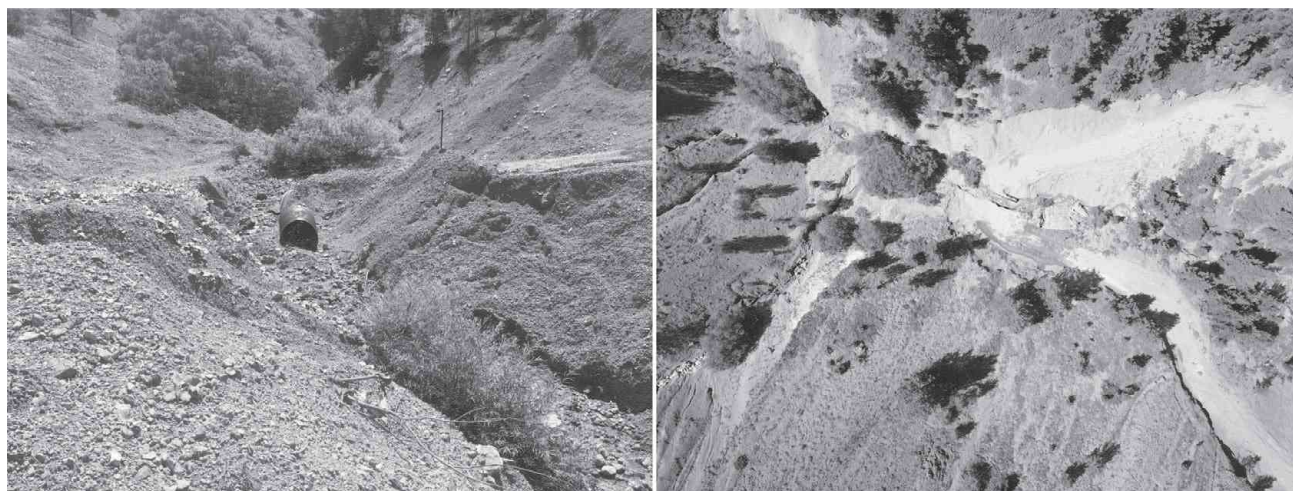
Fig. 4 Deformation due to insufficient CSA of Culvert 15
