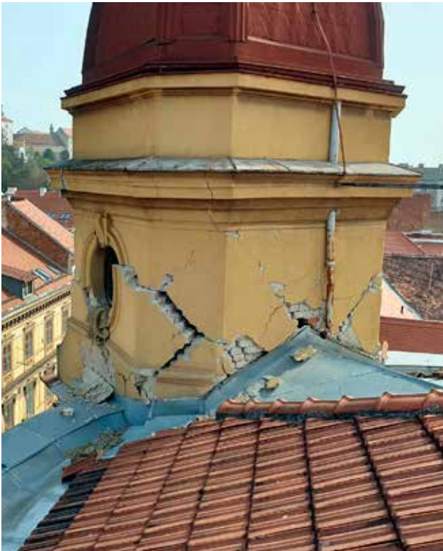
15 Toranj napuknut u potresu, travanj 2020. (foto: M. Todorić) The tower cracked in the earthquake, April 2020 (photo: M. Todorić)
