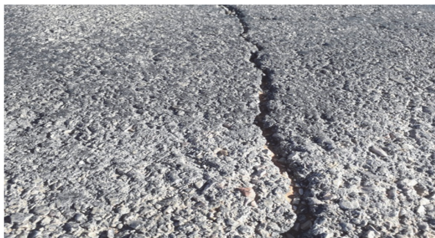
Figure 1 Rise and propagation of cracks on the road pavement
