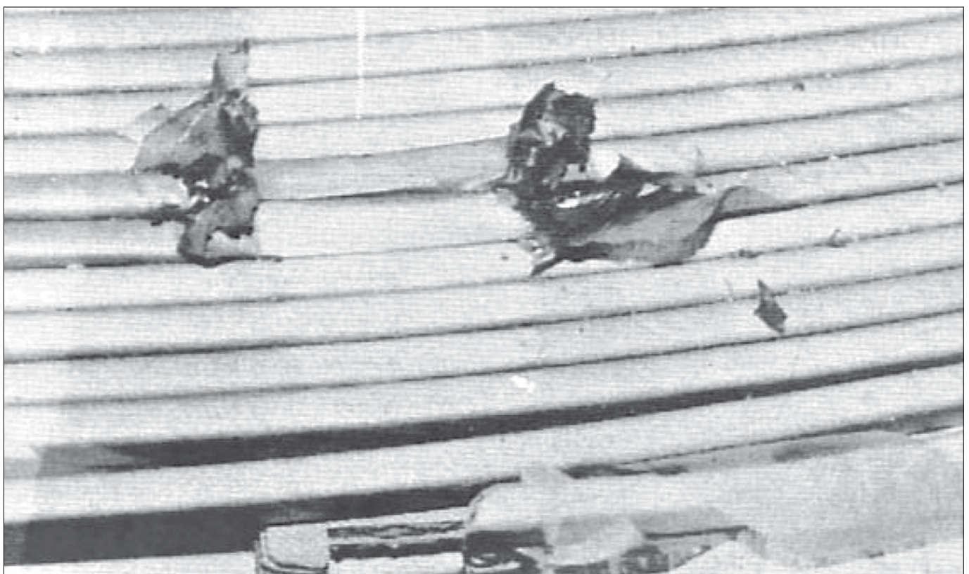
Figure 6. Turn-to-turn punctures found in the discs adjacent to the site of the fault of the main insulation [13]
