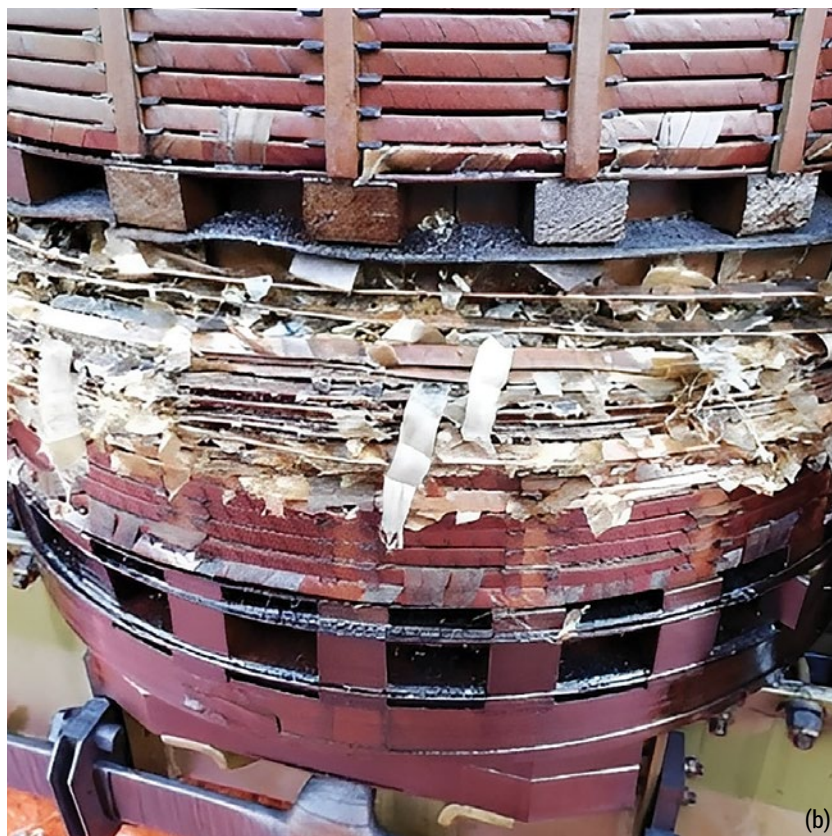
Figure 1.1. (a) Damaged on-load tap changer and (b) damaged B phase of HV winding
