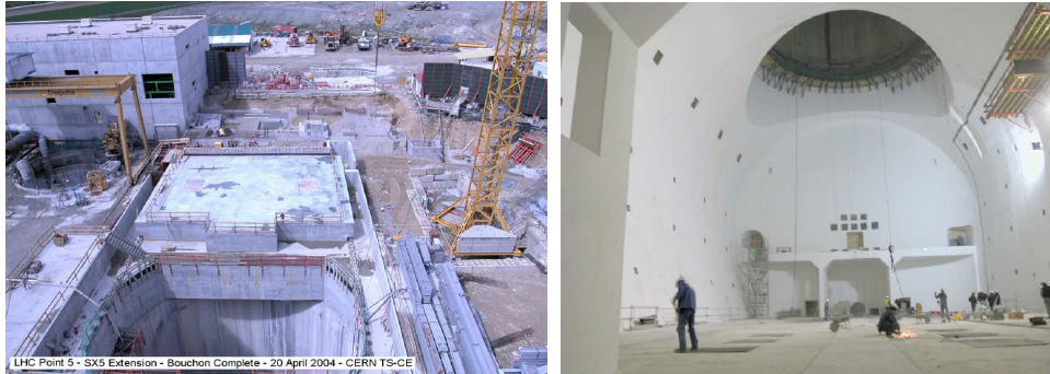
Fig. 2 (left). LHC point 5, with the 24 m diameter shaft to the CMS underground experimental hall and the cover.
