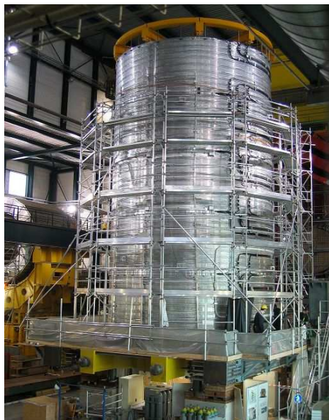
Fig. 10. Five coil modules connected together in CMS surface experimental hall, spring 2005.
