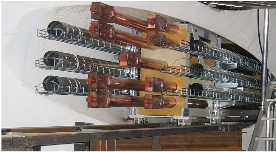
Fig. 11. Passage of the 20 kA bus bars feeding the solenoid through the pillar wall.
