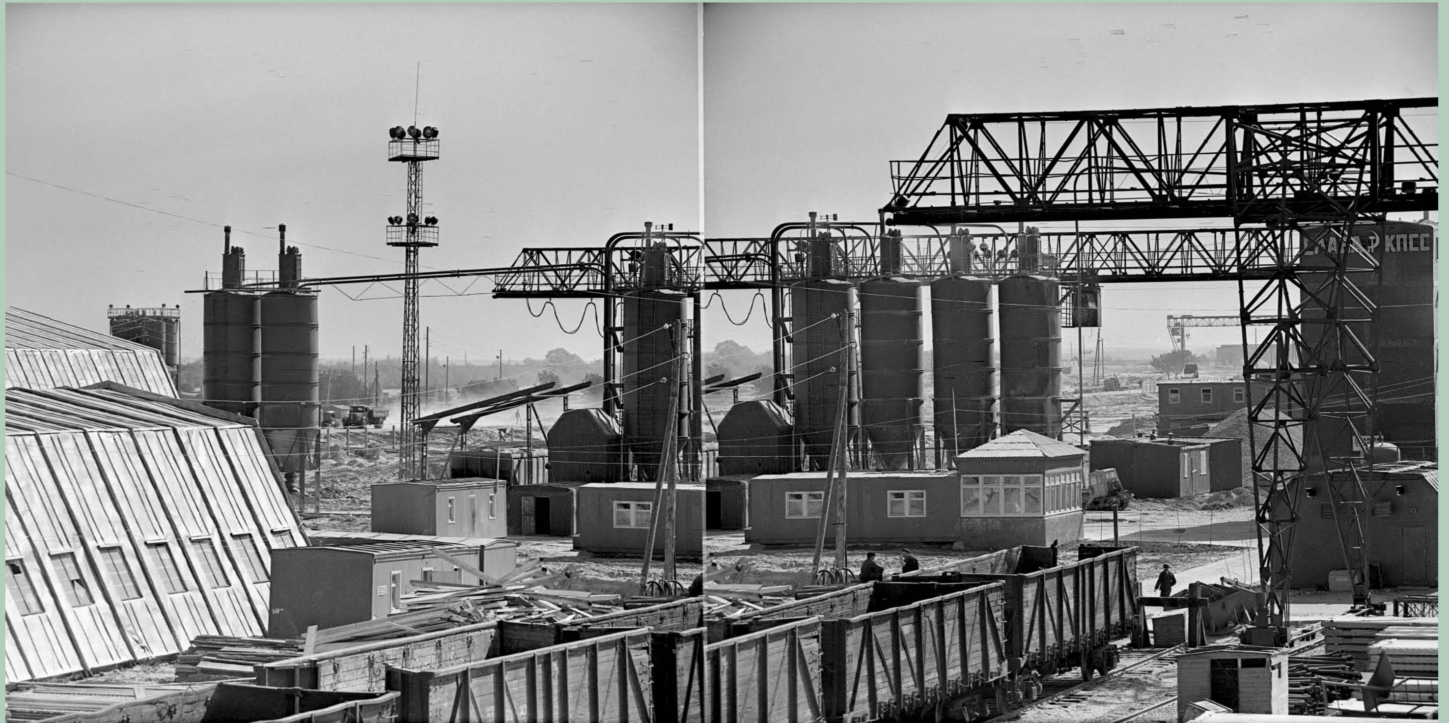
Sl. / Fig. 2 Izgradnja nuklearne elektrane u Chernobylu / Construction of the Chernobyl Nuclear Power Plant, 1971. FOTO/PHOTO: Iryna Pap © Iryna Pap Estate ↑
