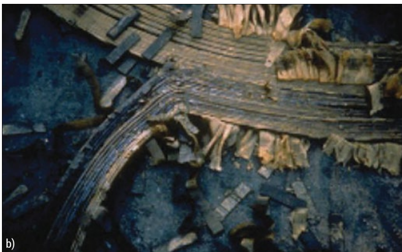
Figure 1. Damaged transformer at the Salem Nuclear Plant. The insulation burned, and the 24 kV LV winding rated for 3000 A melted [1].
