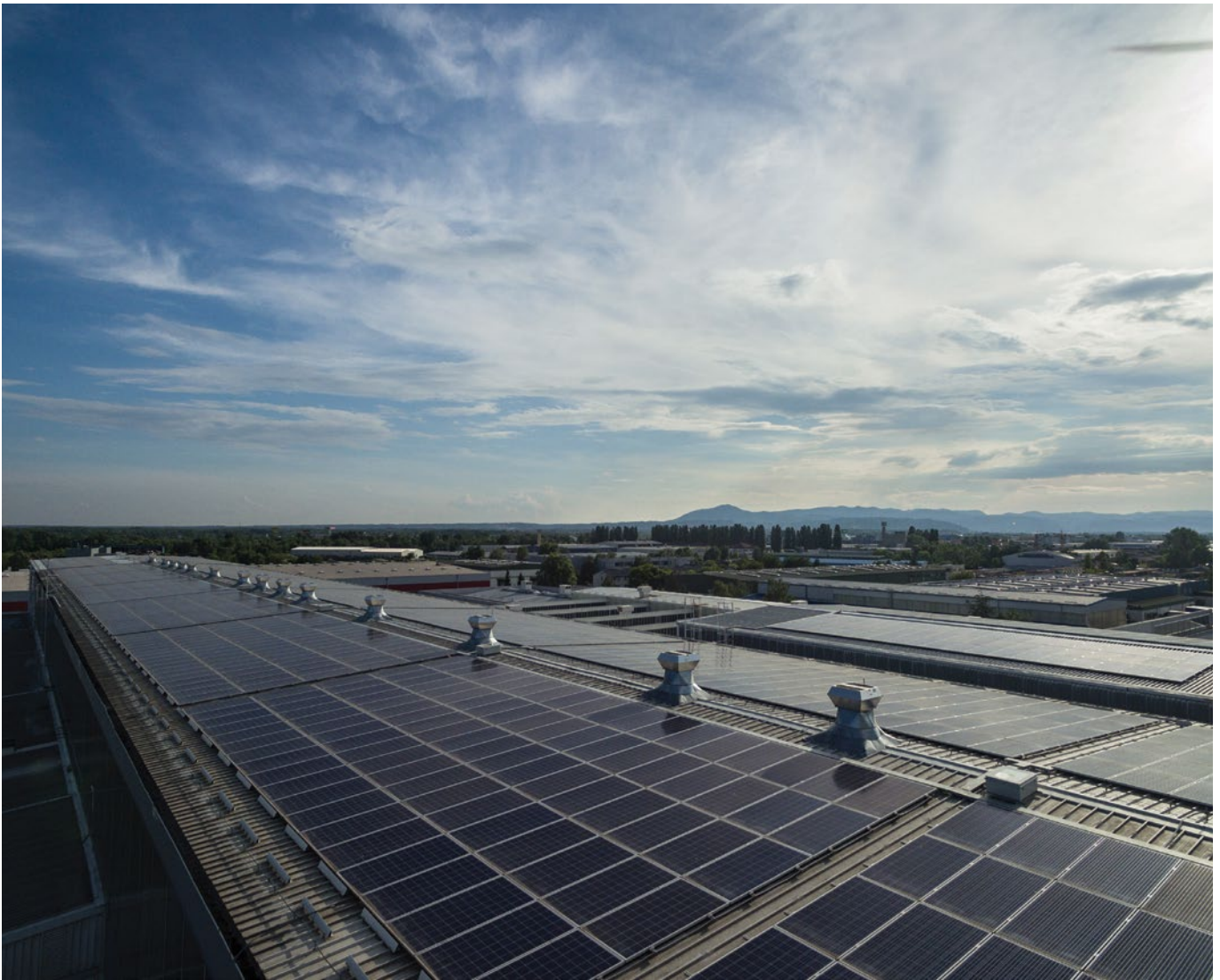
Figure 3. Photovoltaic panels on the roof of the transformer factory in Zagreb, Croatia
