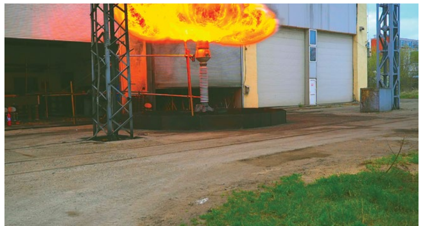
Figure 8. 170 kV CTs internal arc (from top to bottom: mineral oil, MDEL 7131, BIO 300X filled unit)
